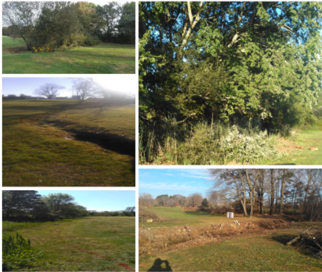
Restoration of Drainage Ditch Hole 4 & 6 & 16 Overgrown and limiting drainage flow Clearing the brush and trees around the irrigation pond
